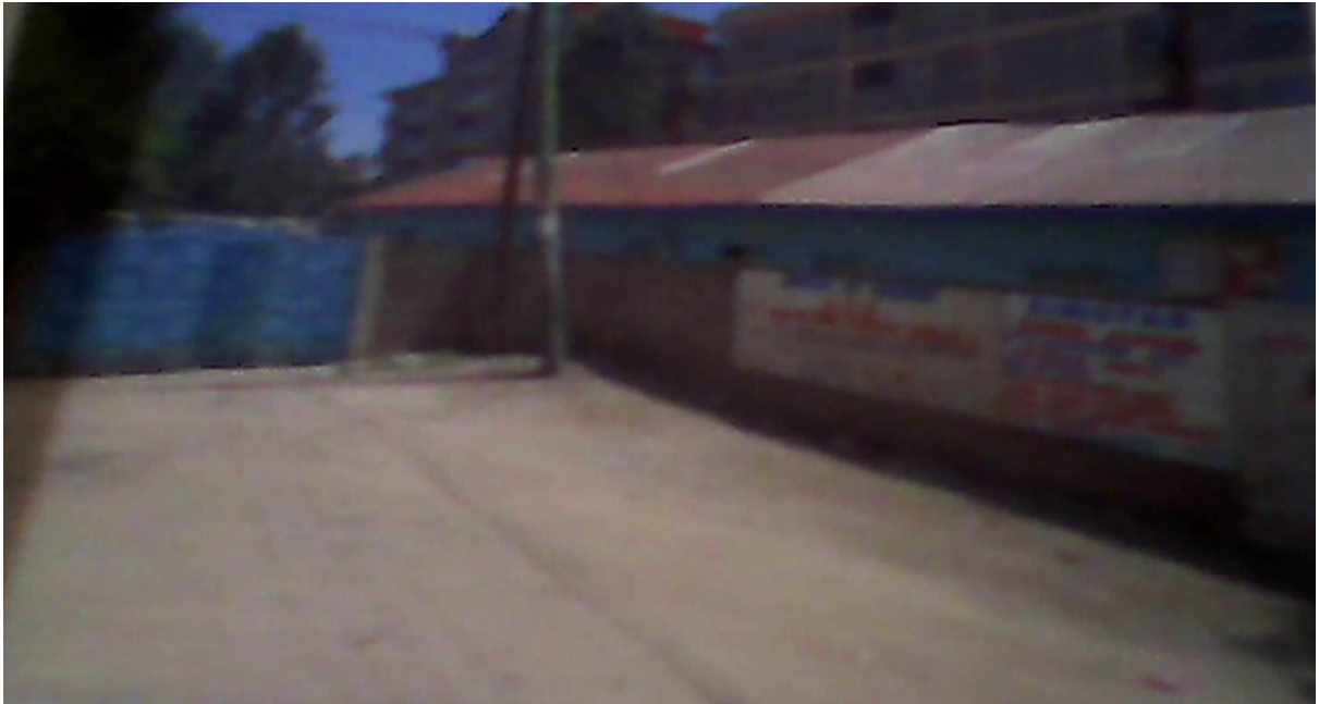
The extension of our church can be seen on the new roof from outside the gate.
